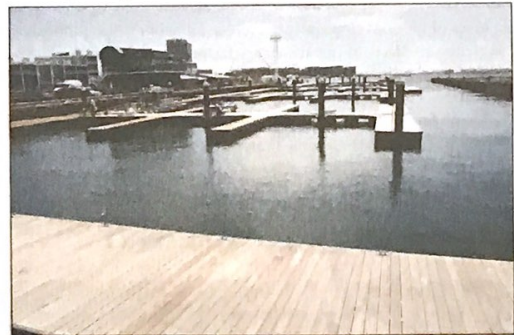
Workers are finally putting the new Pier 6 marina together after more than four years of permitting nightmares for owners Chuck and Ann Lagasse, of the Charlestown Marina. Former owner Martin Oliner created a horrific situation that led to the Attorney General stepping in to sort it out, with the Lagasses taking ownership and having to wait it out with extensive permitting and legal issues brought on by the takeover. Now, however, they hope to have the 100-slip marina expansion operating in August.
